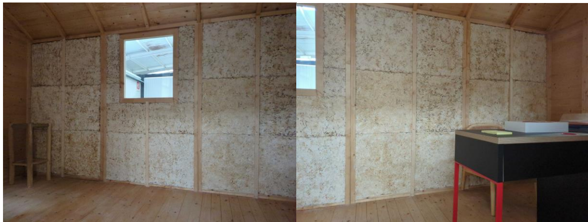
Fig 7. LD panels (low density – prototype 2) being applied on the wall. With application we could also see these were the best examples, as they were lighter and easy to apply.
